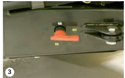
Main switch – OFF
