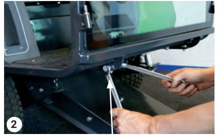
Bolts under base plate
