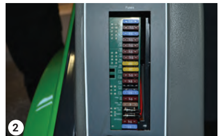
Fuses – cabin floor right side
