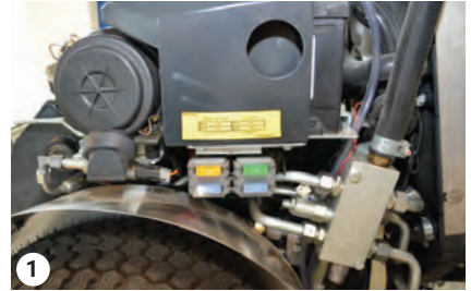
60 A JF15 generator - 60 A JF1 supply fuse box 20 A JF2 emergency line - 30 A JF3 engine power
