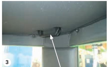
Roof hatch handle
