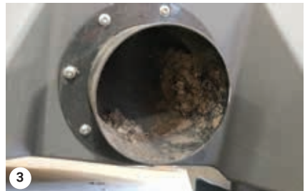
Inlet through the water tank
