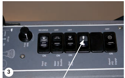
Switch F2, locked position
