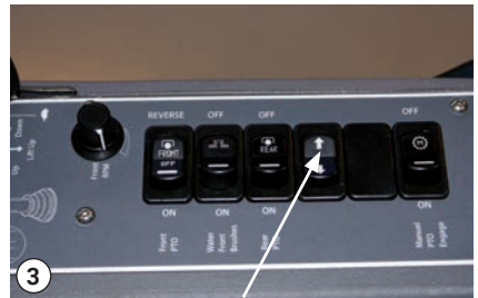
Switch F2, locked position
