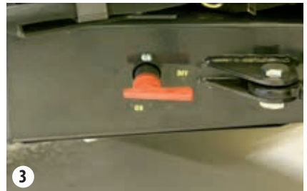
3 Interruptor principal - APAGADO
