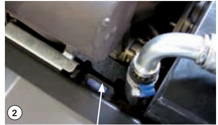
Fusible principal (60 A)
